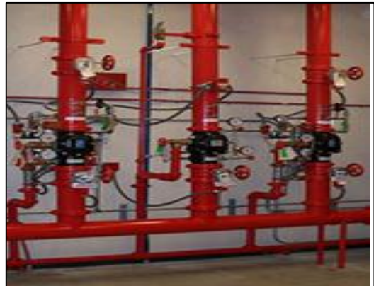
Figure 1. The example of sprinkler system installation realization [1]
