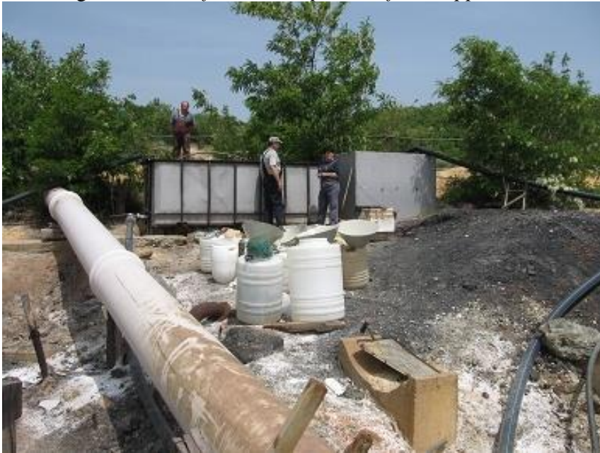
Figure 1: Tanks for the acceptance of the copper mine waters
